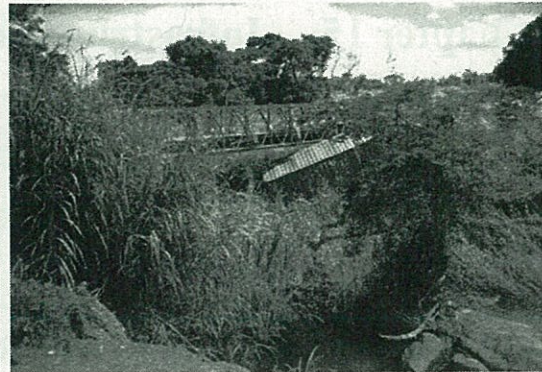
Source: Photo by JICA Study Team Photo 15.1.3. Rolled Truck at Narrow Bridge (R658)
